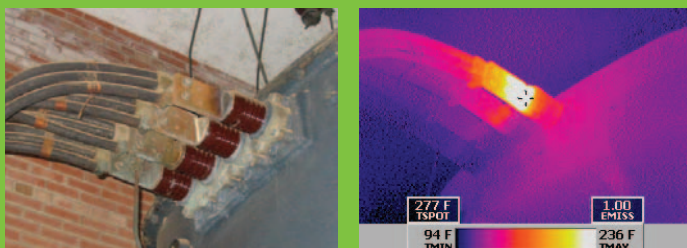
At 94 °F (34°C), one of the terminals on this 1320 V – 480 V main transformer is running hotter than it should.
