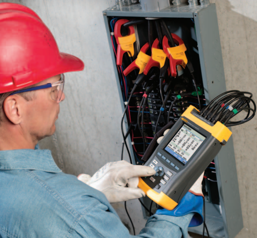
Periodically examine power quality for voltage sags, harmonics and other causes of overheating.
